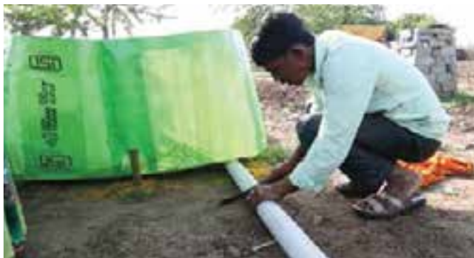
A pipe is fitted at one end for vermi tea outflow
